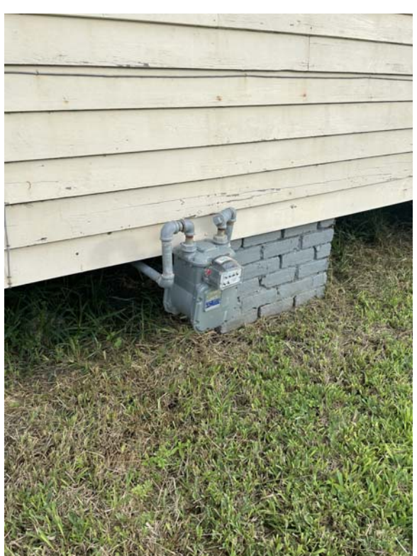
Gas meter connection 2
