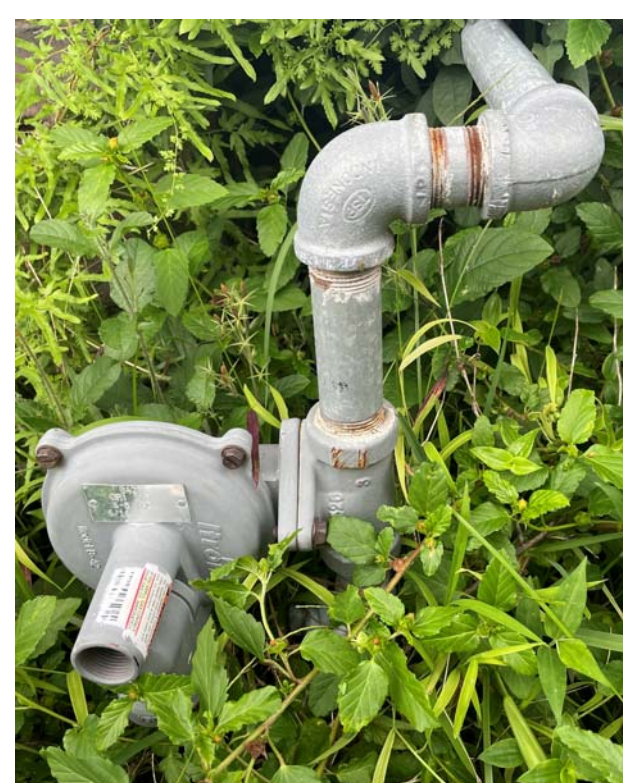
Gas meter connection 1
