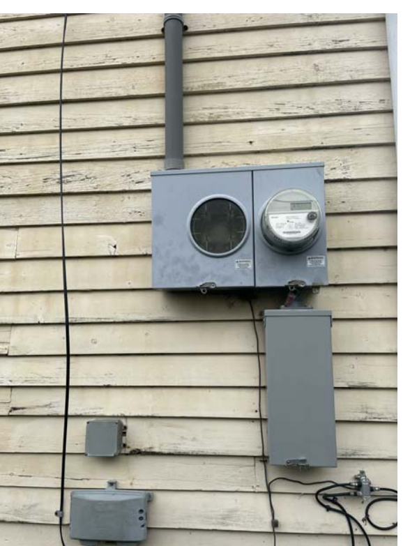
Existing electric meters for two units
