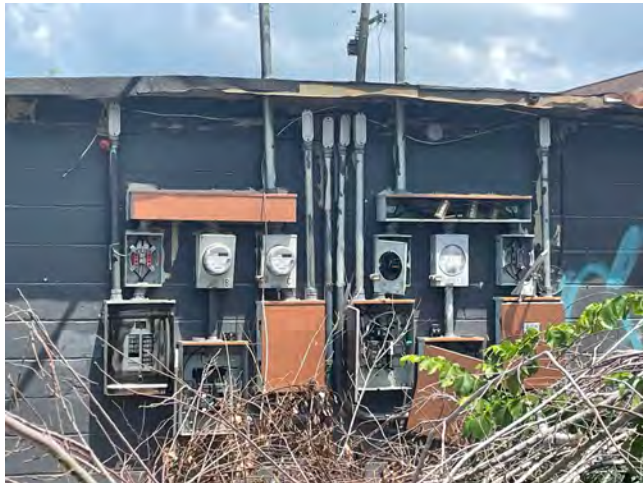
Dangerously exposed wires and again only two functioning electric meters. Photo taken 6/17/22.
