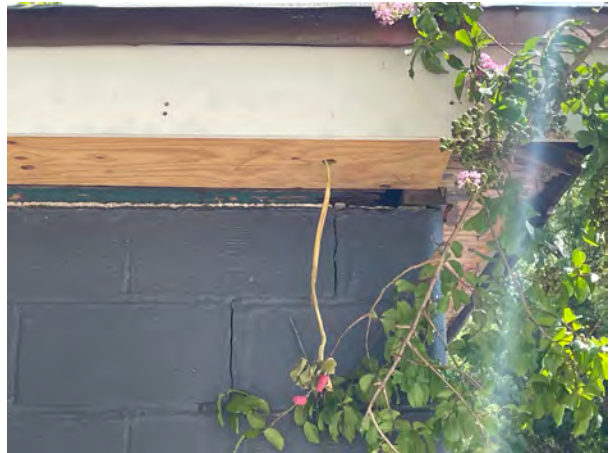
Cracked structural walls and rotten top plate next to new eave and fascia. Photo taken 6/17/22.
