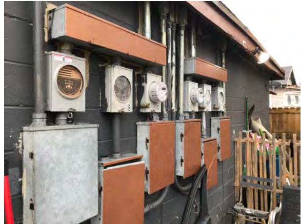
Only two functional electrical meters. Photo taken on 2/5/2021.
