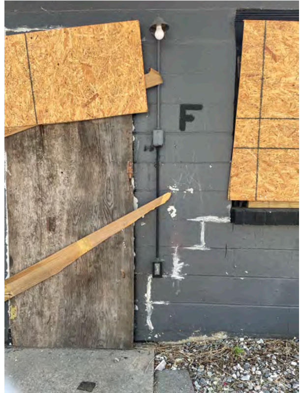
Cracked structural walls attempted to be fixed with caulk. Photo taken 6/17/22.
