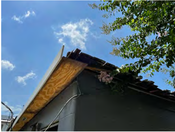
New eave and fascia covering up rotten roof. Photo taken 6/17/22.
