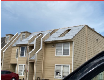
BUILDING 17: shingle overlay left and right end of building penetrated with cap nails and synthetic. approx 50% of mansard roof area at front
